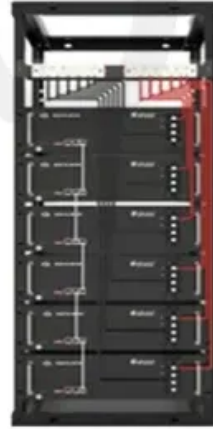
Cabinet and rack installation display
